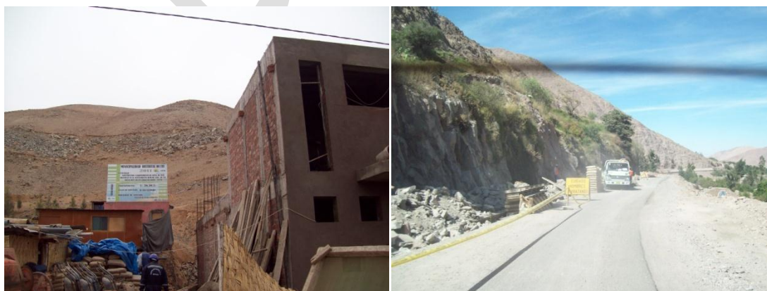
Municipal construction Project about to start in Ite (left) and road construction in Torata (right)
